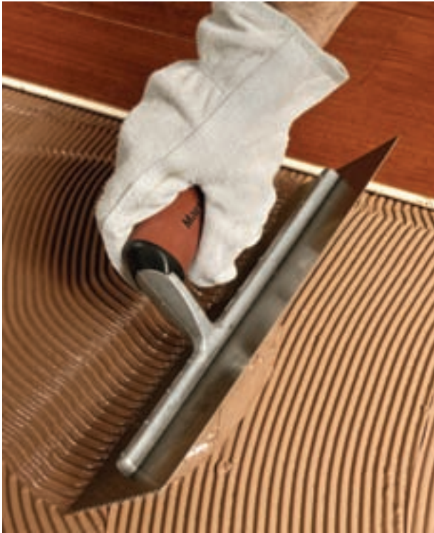
When most people hear of moisture related problems they usually think the flooring product is either carpet or resilient but wood can be just as if not more susceptible due to its nature to absorb water. That is why companies like Bostik have created adhesives, such as its Vapor-Lock line, that are designed to protect the wood flooring.
