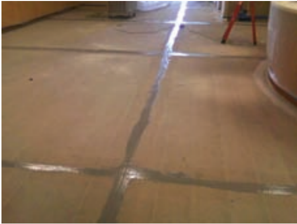
Some of the many aspects of moisture mitigation contractors such as those like Resource Arizona do is using epoxy in the joints and shot blasting the floor to remove the emulsified adhesive and to open the pores in the concrete to prepare it for the next step.
