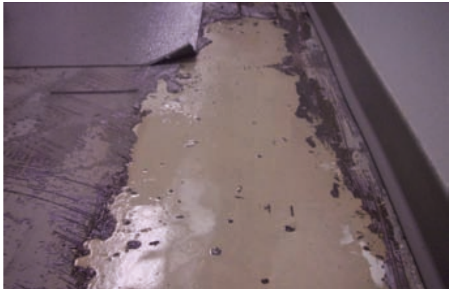
Sometimes you don’t know exactly how bad a moisture/water problem truly is until the flooring is taken up and the results can sometimes be troubling as seen here.
