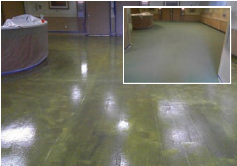
While many people around the country will think places such as Arizona are not as susceptible to moisture related problems, the folks at Resource Arizona in Phoenix will beg to differ as their crews had to prep this floor—and room—to help solve a difficult moisture problem. As the after photo shows they were able to mitigate the issue and had the subfloor ready to receive the actual floor covering.
