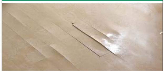
Figure 1. Moisture and pH problems led to strip failure, stressed vinyl composition tile and efflorescence in the seams.
